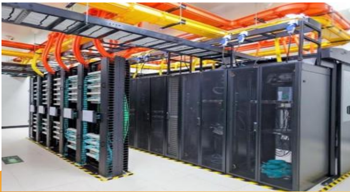
6 500 nodes of CAT.6A FTP Solution and around 10 000 OM 4 ports for The Data Center of PolyU.
